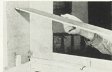
Insert puppet floor, which is a 5" shelf. Holding it in place, drill two holes through it into the wooden blocks. Turn in wood screws and cut off heads, leaving short pins. Hold shelf with hooks to front and wing blocks.
